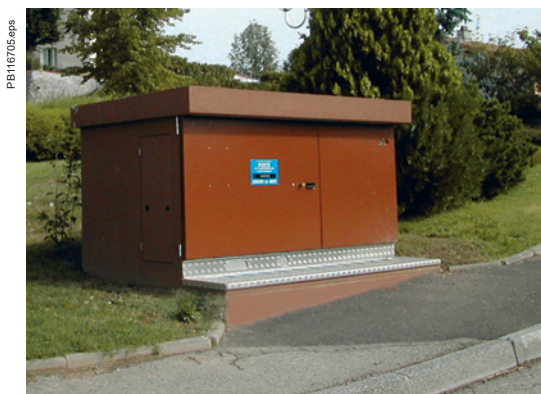
(b) Half buried non walk in type substation
