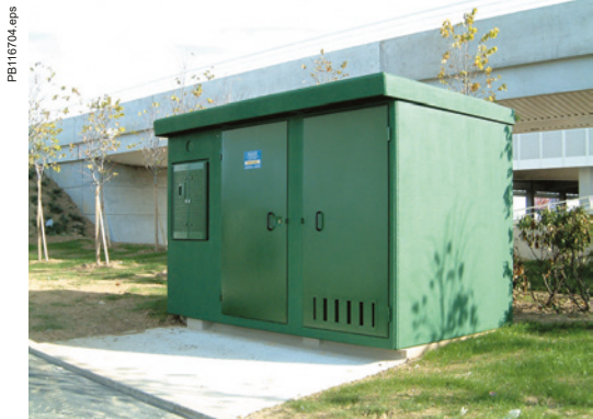
(a) Ground level walk in type substation
