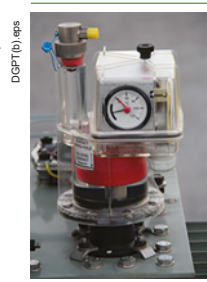
(a) Transformer protection relay (DGPT)
