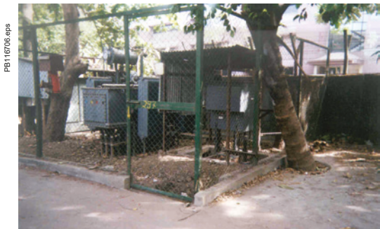
Fig. B53 Outdoor substation without enclosure
